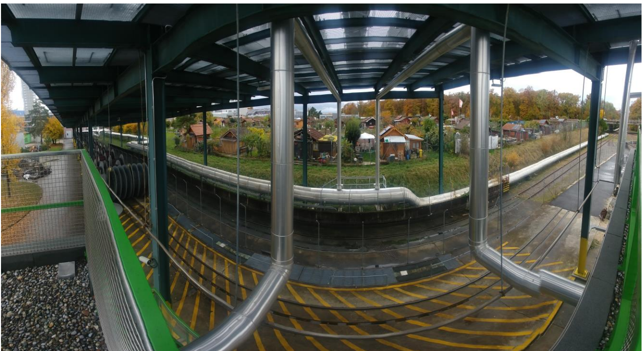
The solar thermal installation SolarCAD II of Geneva Industrial Services (SIG). Photo: Verenum AG (Stefan Thalmann)
